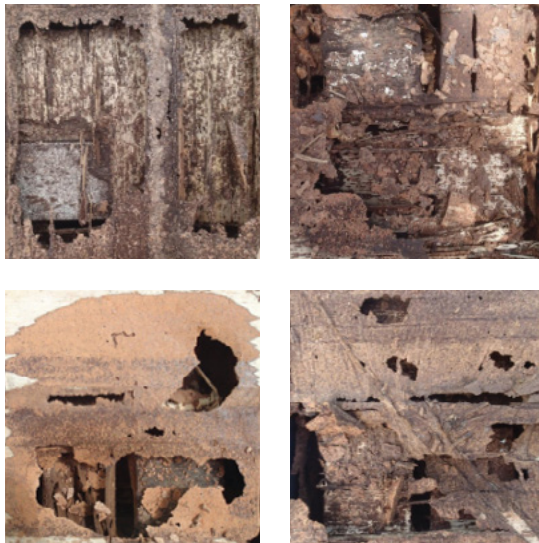
○ Internal termite damage – untreated Pine.
