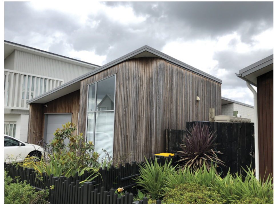
○ Uneven weathering of uncoated Western Red Cedar.
